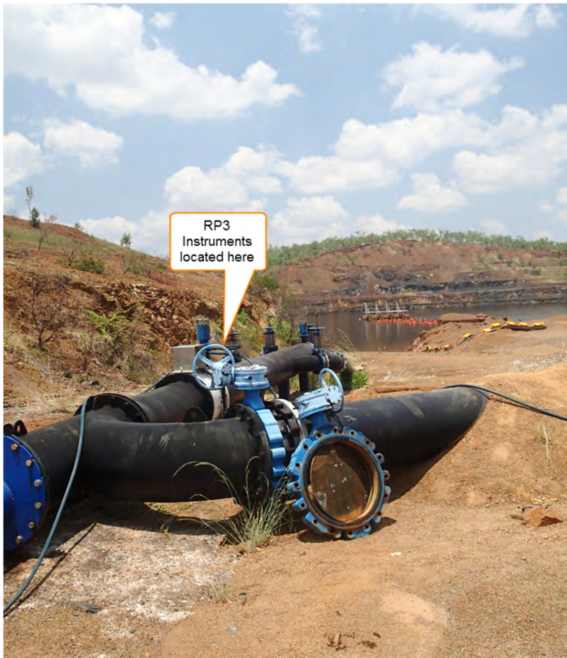
Figure 3-1 Batman Pit in-line water quality monitor
