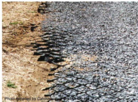
Plate 3-2 An example of cellular confinement system used to retain soil and assist in the establishment of grass
