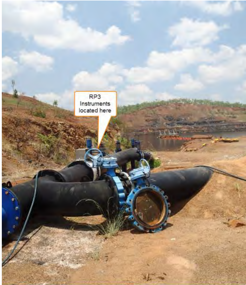
Figure 2-9 Batman Pit in-line water quality monitor
